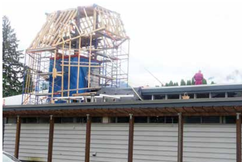
Bishop John on the roof prior to worship, the work area is visible on the left. PHOTO Randy Murray
